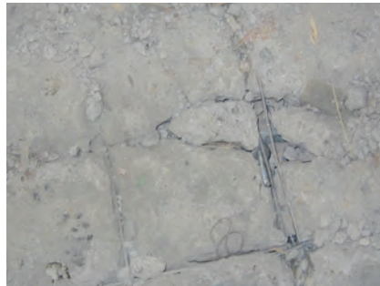
Cracked and Spalling Concrete
