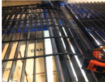
Damaged Bar Grate
