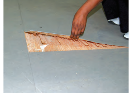
Damaged Poly Deck
