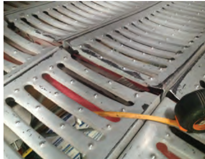
Damaged Plank Grate
