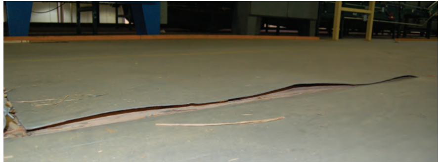
Damaged Poly Deck
