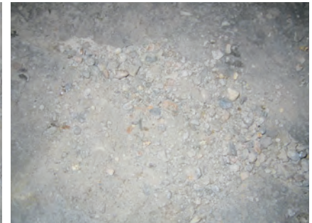
Cracked and Spalling Concrete
