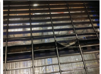
Damaged Bar Grate
