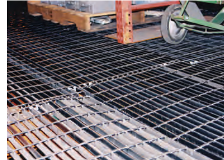
Damaged Bar Grate
